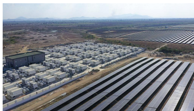
Figure 6: Solar PV and battery storage at the National Solar Park in Kampong Chhnang, Cambodia
