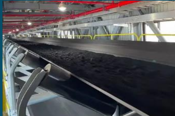
Open Belt Conveyor
