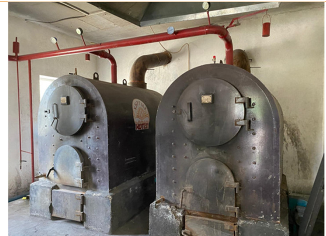
Existing coal-fired boilers in a targeted school
