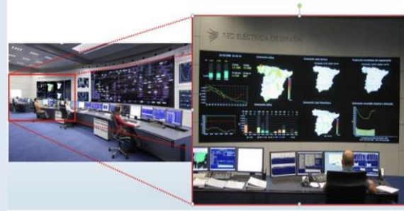
(CERCE, RE Control Room in Madrid)
