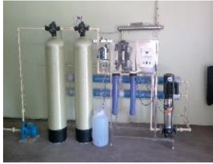
Water Treatment Unit
