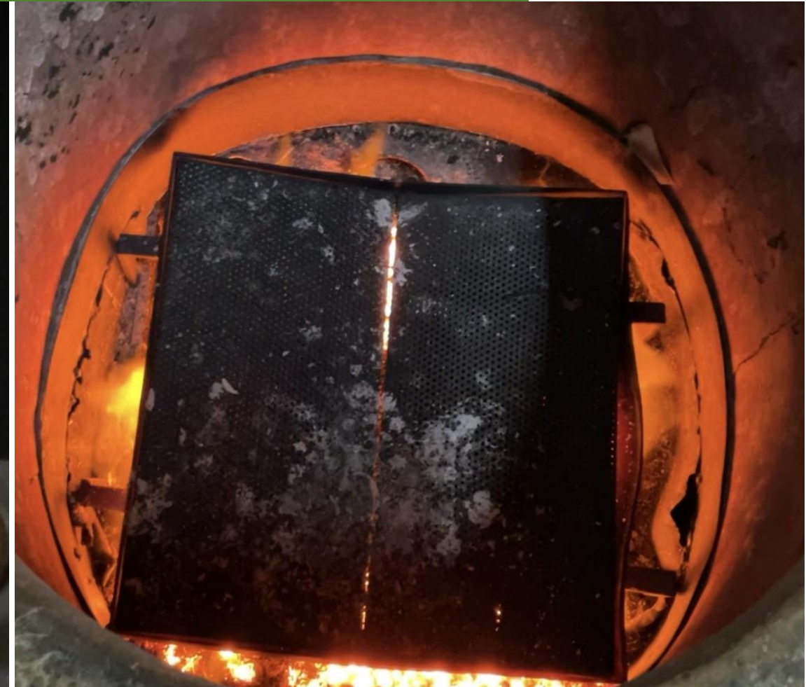
"Coal to Biogas fired Tandoor (~35% Coal saving & 50% faster)
