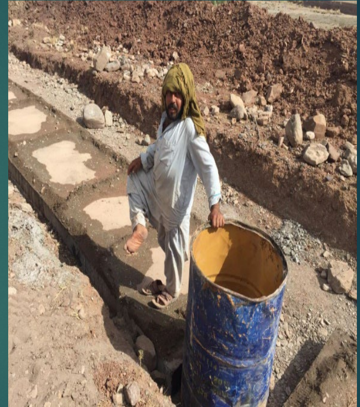
Worker with no safety boot and wound on feet
