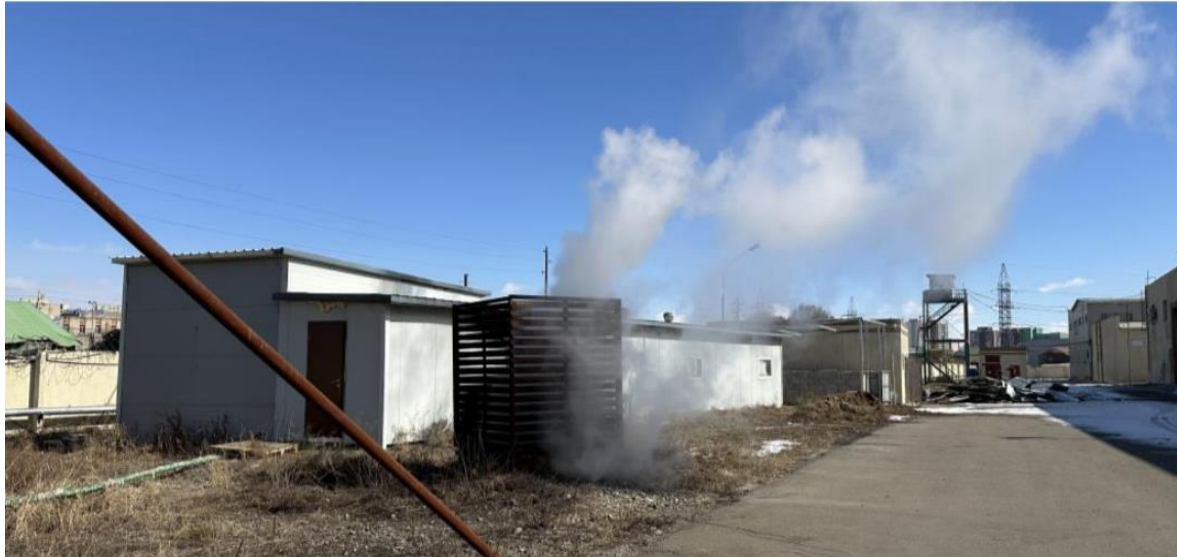
Company's current wastewater treatment plant, 2024
