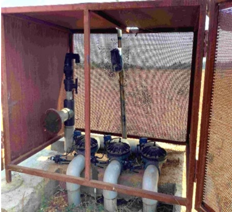
Control Hub: air valve and flow and pressure control to 75 ha units with remote SCADA monitoring & actuation
