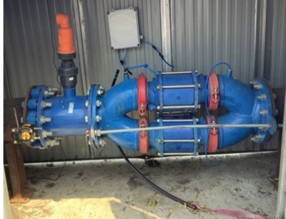
Control Hub (remote management system) with air valve, air flow and pressure control to 250-300 ha units with remote SCADA monitoring
