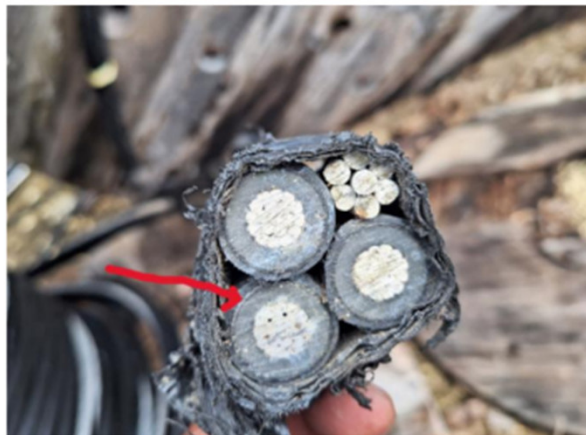
Figure 4 – ABC conductor found at the TPL yard left over stock with red arrow pointing to the metallic sheath surrounding the insulated area.
