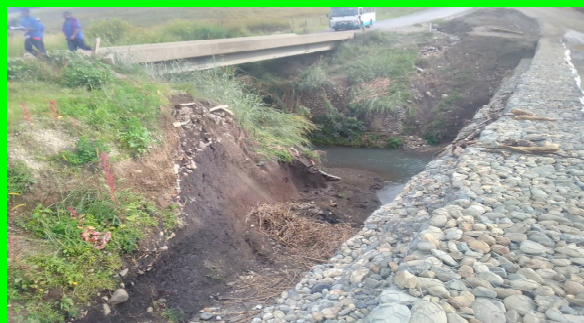
UNSAFE WASH BAYS AND ACCESS
