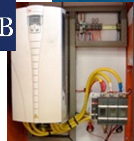
Example of VSD
