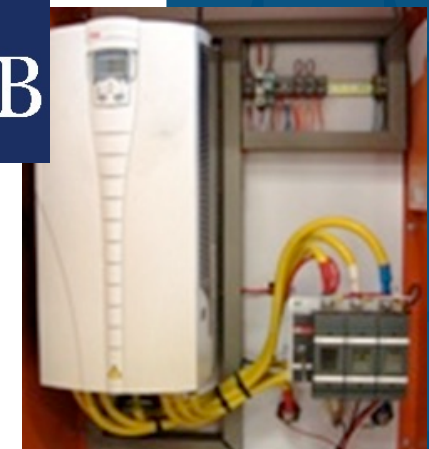
Example of VSD
