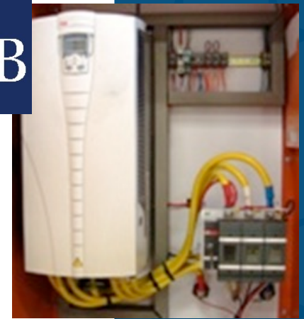
Example of VSD
