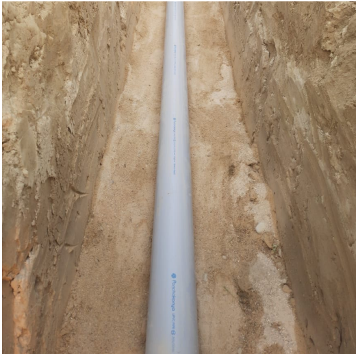
Buried pipe distribution system
