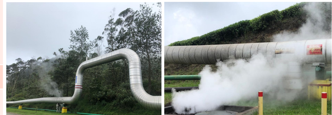
Geothermal steam pipes
