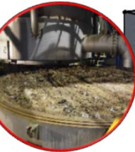
Bottom Ash Conveyor
