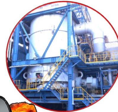
Low-temperature Pyrolysis Gasification Furnace
