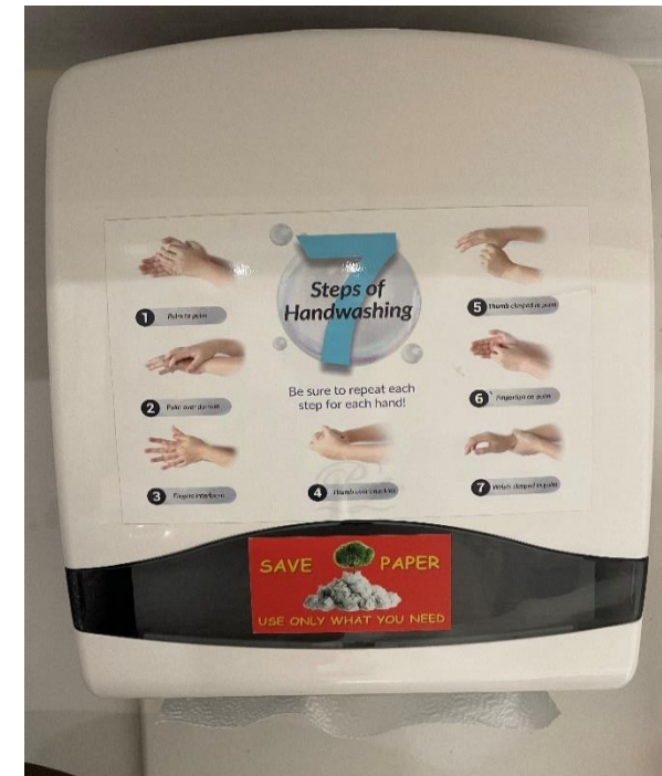
Dispenser at toilets
