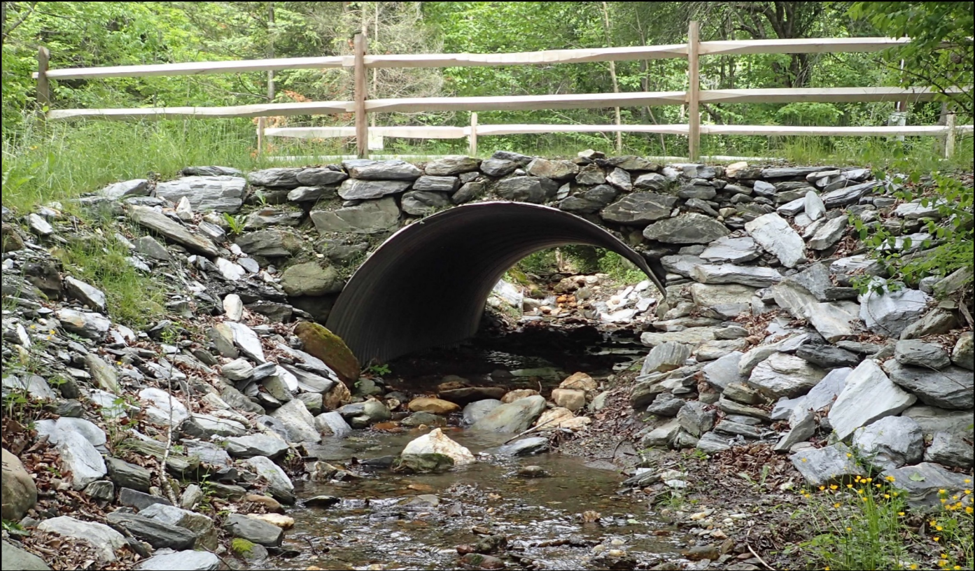
Hurricane Irene: 1000 traditional culverts damaged, none of the stream simulation ones were
