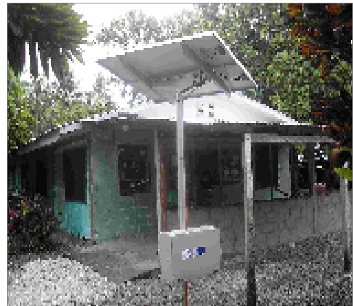
Household solar PV system Installed at Jeh, Ailinglaplap Atoll
