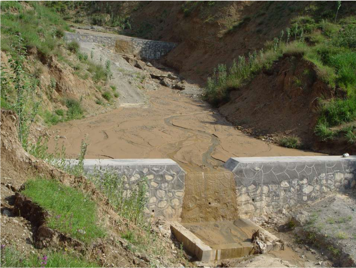
Onsite Monitoring Station
