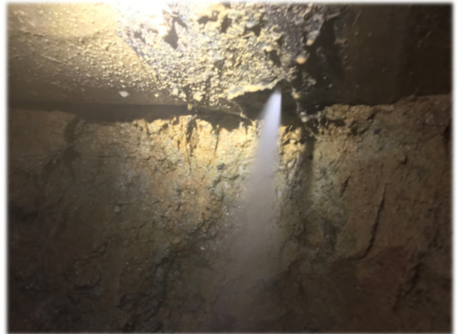
Pinhole leak at point of interest
