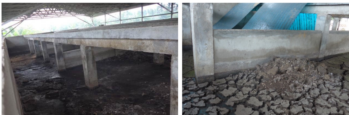
Figure 17: Sludge Drying Beds
