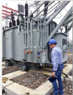
Safeguards Site Visit to Kualanamo and Galang Sub Station-North Sumatra 31 st October 2018
