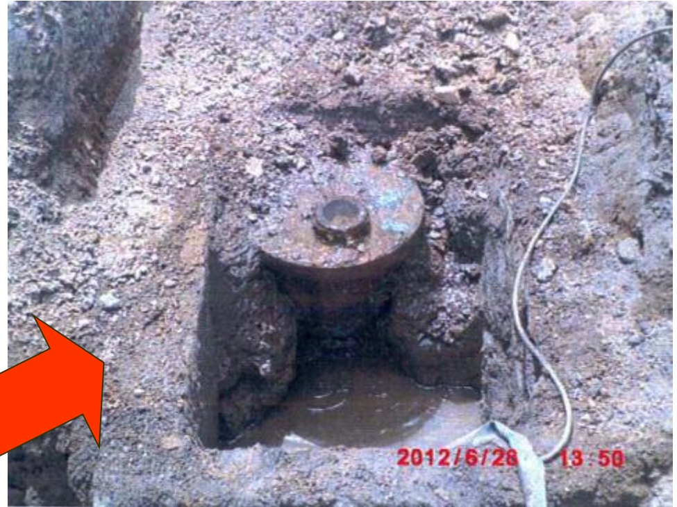
a leaking exhaust valve
