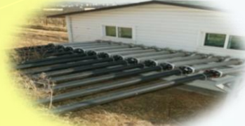
Manifold Station for Gas Transmission
