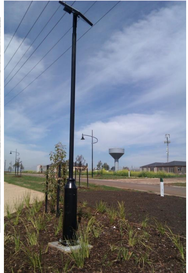
Solar powered impressed current
