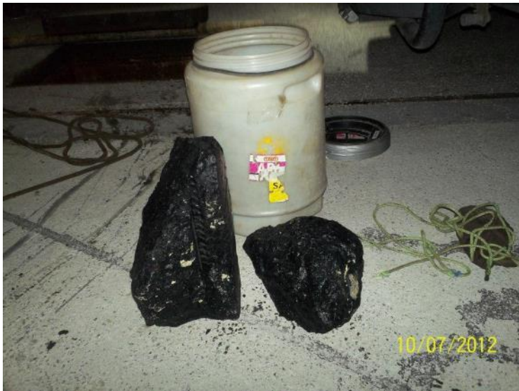
Debris removed from Dudley Street sewer
