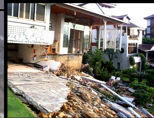
Potential fault rupture
