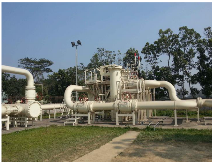
Figure 3: Monohordi Gas Metering and Manifold Station. Photo taken during field visit on 14/02/2013
