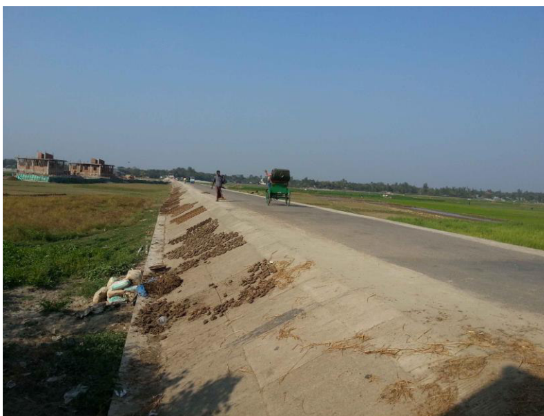
Figure 4: Approach road of Panthasala bridge constructed on Meghna river flood plain. Photo taken during field visit on 20/02/2013
