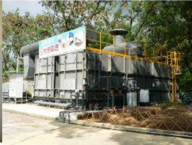
Deodourisation of compost produced gases
