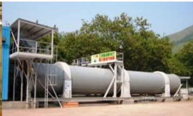
Rotary in-vessel composteer where bio-degradation takes place
