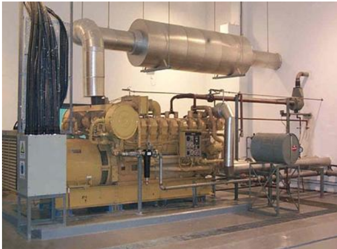
Power Generation From Landfill Gas
