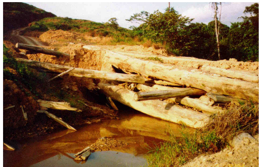
Plate 4.15: A collapsed temporary crossing obstructing a stream channel
