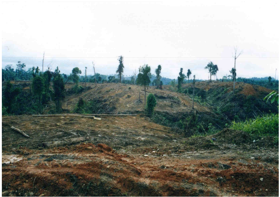
Plate 4.2: Typical site clearing sequence that entails clearing of underbrush followed by felling of tree stands. To reduce ground surface exposure to erosion, the activities may be modified by carrying out tree felling first and followed by spot clearing of under brush along oil palm planting lines
