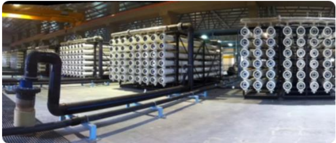
AZE: Reverse Osmosis Plant in Nakhchivan
