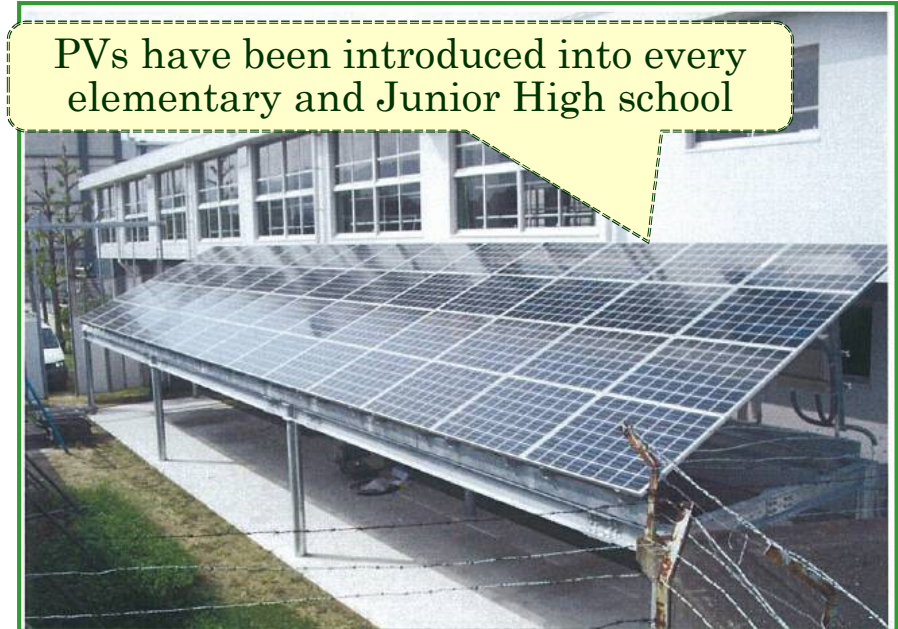
Photovoltaic Generation at School
