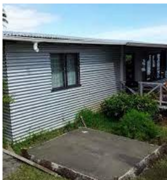
Figure 2 Tank base and gutters installed to meet requirements for the WAF Rainwater Tank (Water Authority Fiji)
