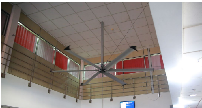
High volume low-speed fan to improve air circulation inside the building
