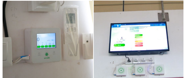
Indoor air quality sensor (left); live display of building indoor air quality and energy data (right)
