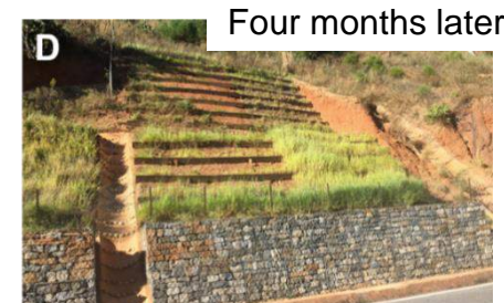
D: After the vegetation works, taken photo on October 31, 2020
