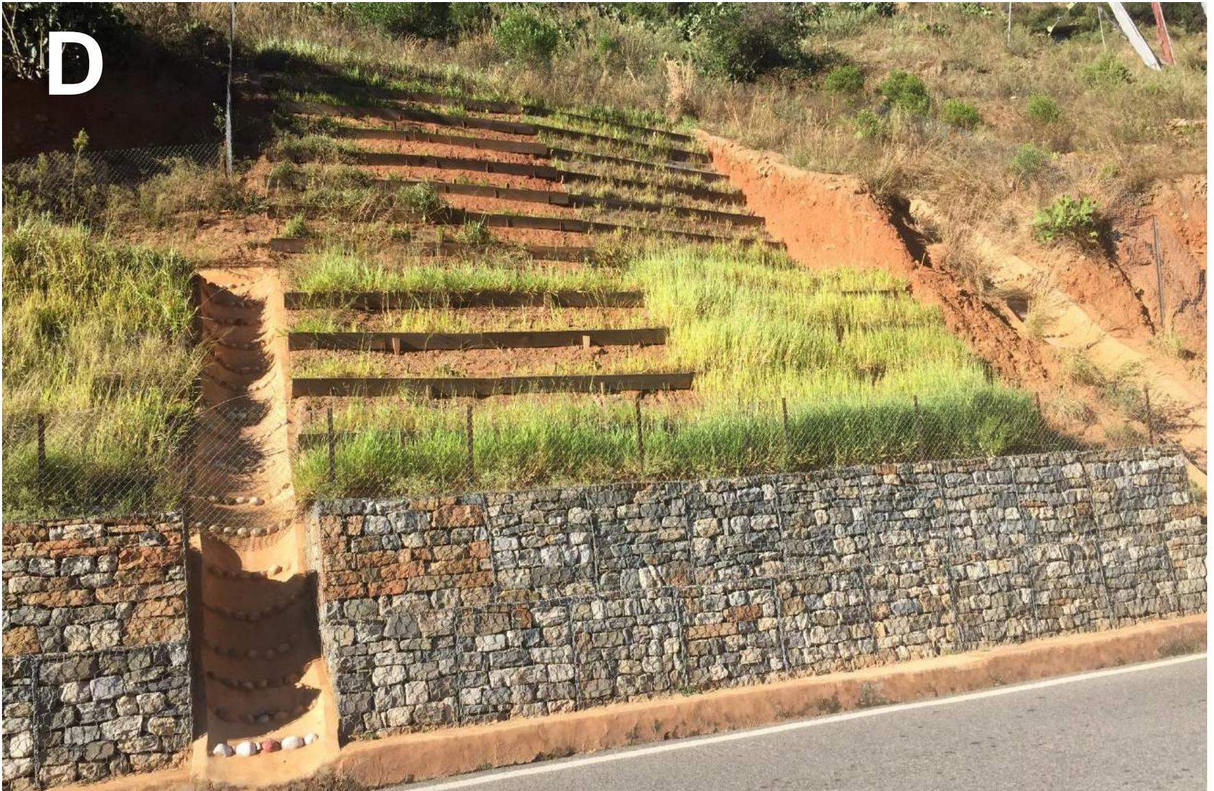
D: After the vegetation works, taken photo on October 31, 2020
